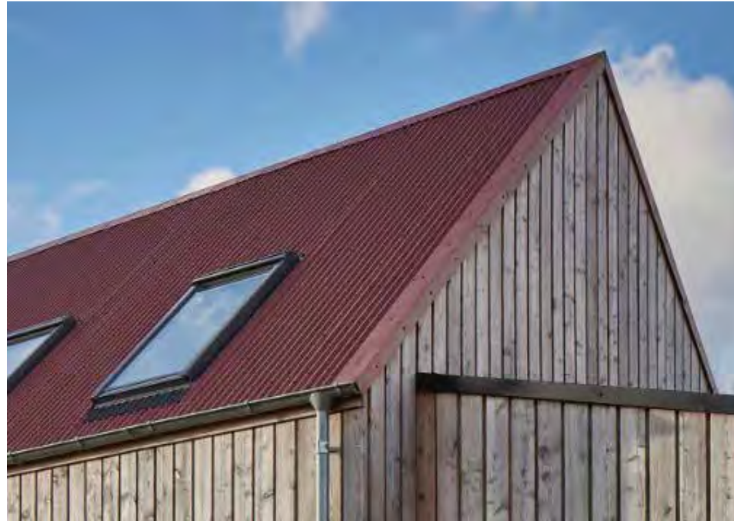
Profile metal roofing and timber cladding is another common combination, often seen on outbuildings and netting sheds. The profile metal can be supplied in a variety of colours from grey through to red.
